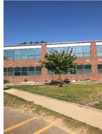
Typical Wall Louvers – Fresh Air and Exhaust Air
