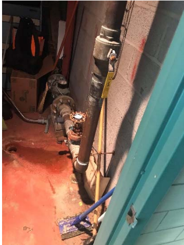
Water Entrance and Water Meter
