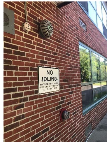
Fire Protection Gong and Hose Connection
