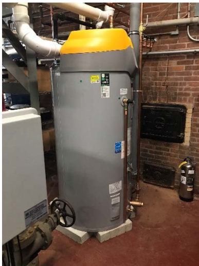
Supplemental Domestic Hot Water Heater
