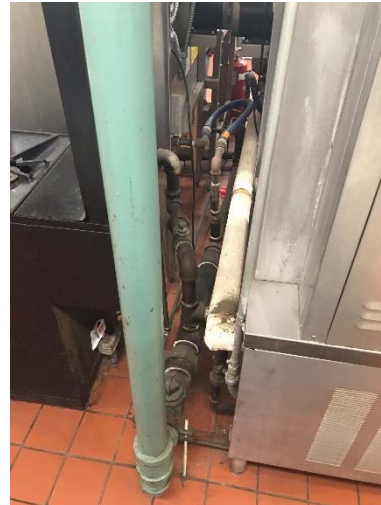
Natural Gas Pipe to Kitchen Appliances
