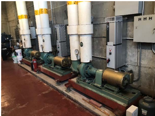
Typical Hot Water Pumps
