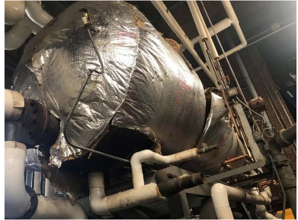
Indirect Hot Water Heater and Storage
