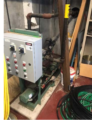
Fuel Oil Pump
