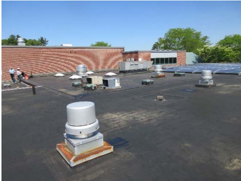
Typical Exhaust Fan
