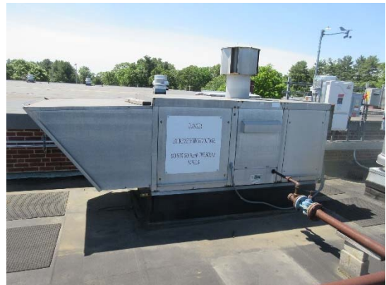
Typical Ventilation Roof Top Unit
